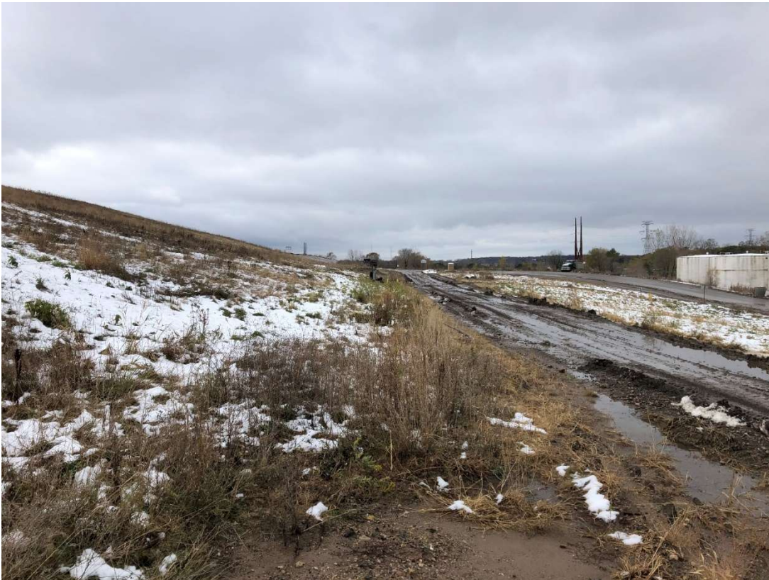
Location 13 – Looking Southwest, Cell 1 Toe of Waste Slope, Limit of Industrial Waste (CCR)
